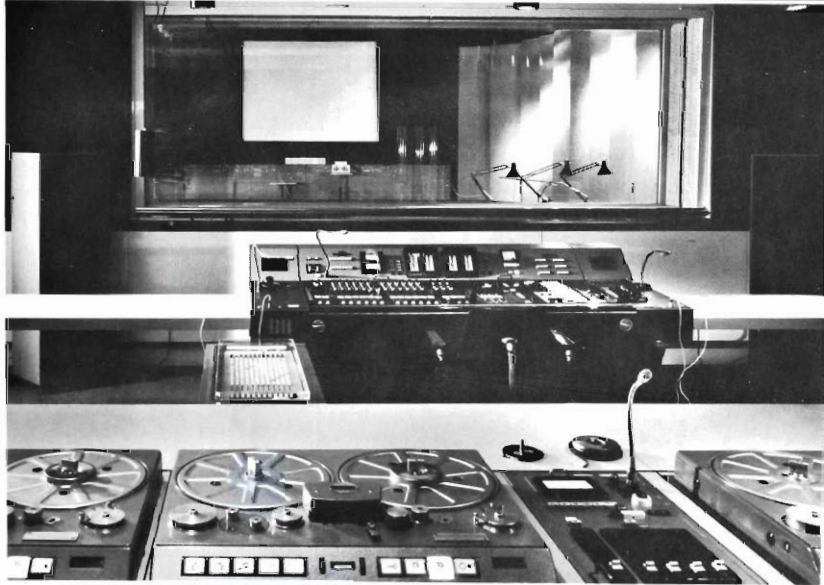
Fig. 29 Looking from the control room of one of the dubbing (synchronizing) studios into the studio proper. ORF uses many films from other countries and its facilities for dubbing new sound tracks on these are very elaborate.
