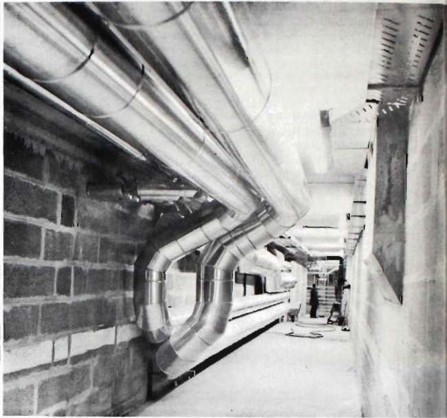
Fig. 31 Heat, air-conditioning, power, hot and cold water, control cables, intercom and telephone circuits, etc. are distributed throughout the complex by a series of "energy canals", such as that shown here, which run like a maze under all the buildings.
