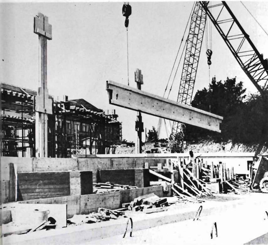
Fig. 10 The reinforced-concrete girders used in the Zentrum Wien buildings are unusually large—being 15 meters (50 ft) long by 1.5 meters (5 ft) high. This size was determined from functional and static considerations.
