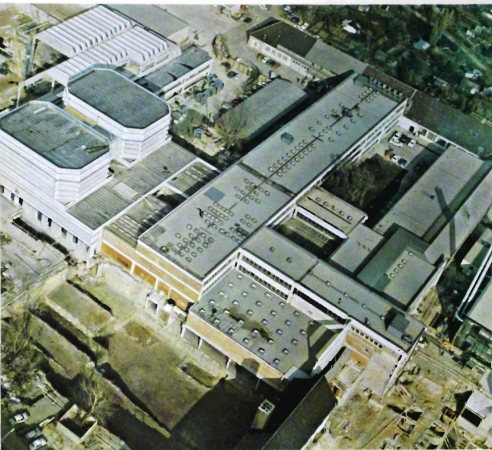
Fig. 19 In this view of the complex under construction, the low building (bottom, center) with the many skylights is the central machine room. The central equipment room and master control area is between the machine room and the studios. The area at the bottom left of this photo is where the main office building will go. From the first floor lobby of the office building the central machine room will be visible thru a larger glass wall.
