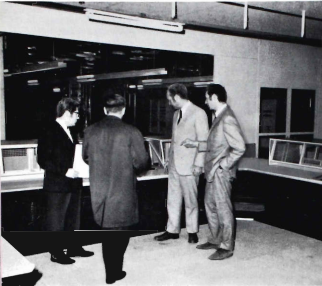
Fig. 23 A view in the master control room during early stages of installation. Operators sitting at the console will face a large group of monitors and read-out displays which will be mounted in the wall opening which can be seen at the rear in this picture.
